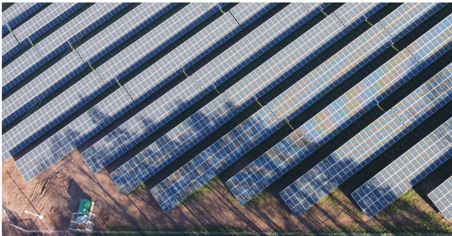
The radar and camera can be seen on the camera pole in the bottom left corner
