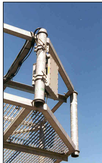
Base Station Transceiver
